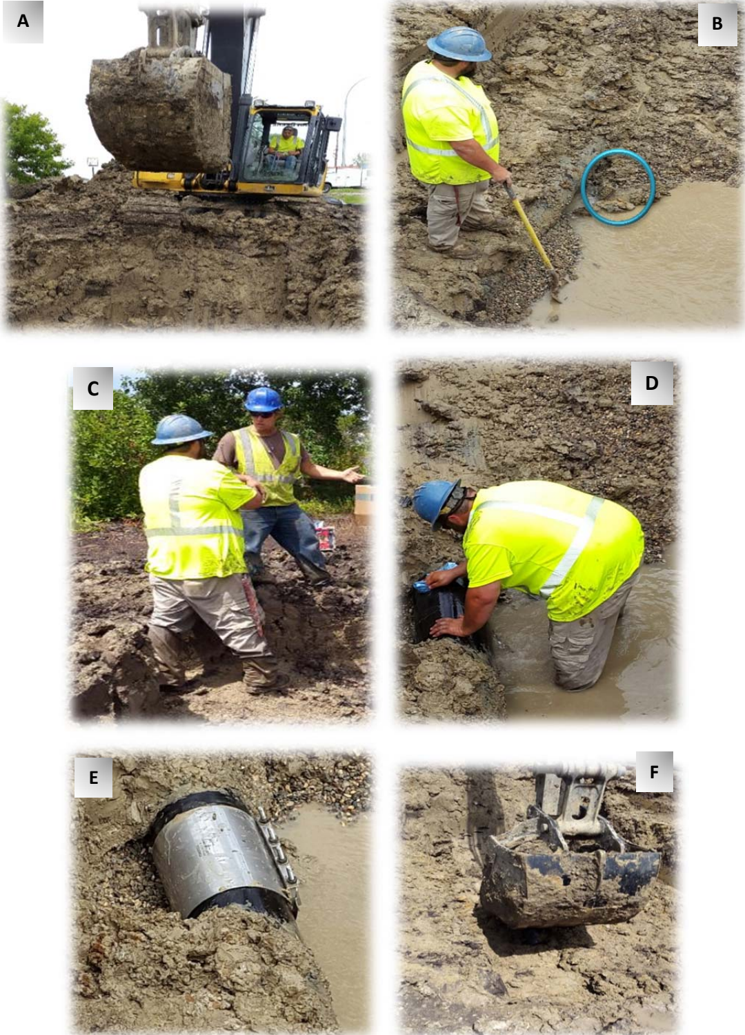
Figure Descriptions: A) Excavation, B) Detection, C) Assessment, D) Pipe surface cleaning for repair, E) Repair, and F) Backfill and pave.
